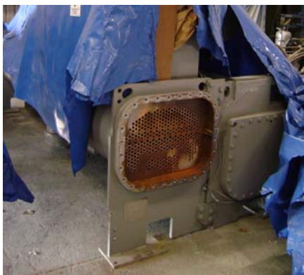
A new chiller exhibits corrosion from its factory testing.
